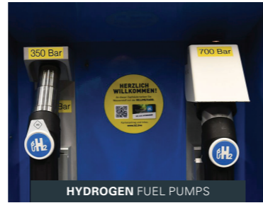
HYDROGEN FUEL PUMPS
