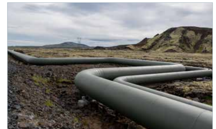
District heating supply
