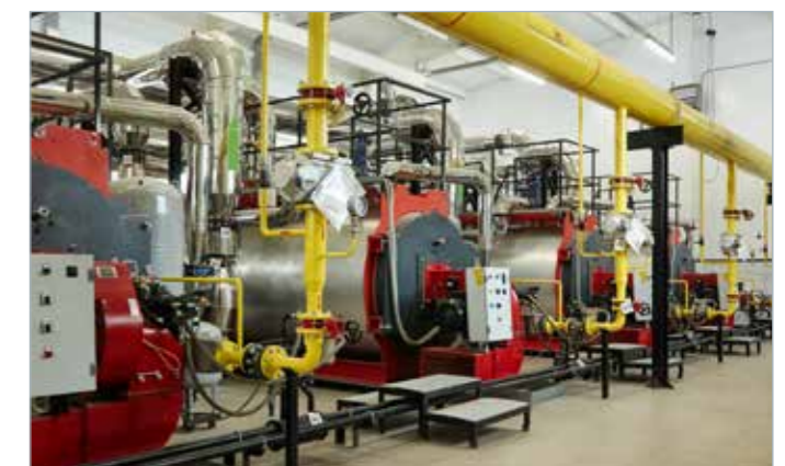
Large-scale heating systems
