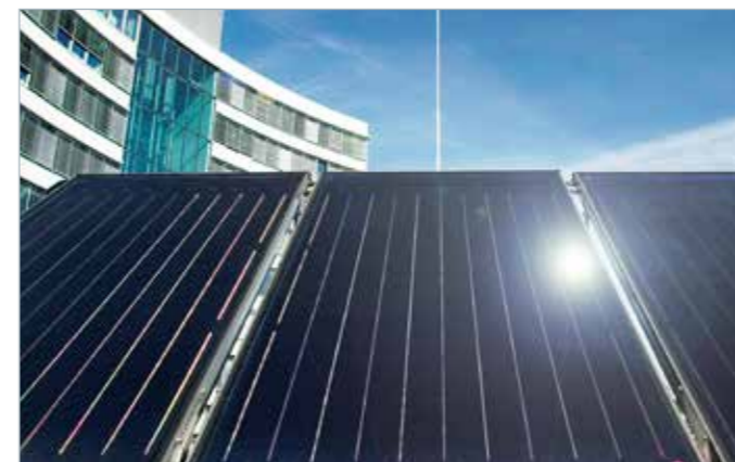
Solar power plants (collectors)
