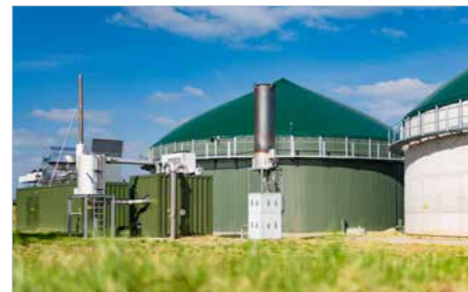
District heating generation
