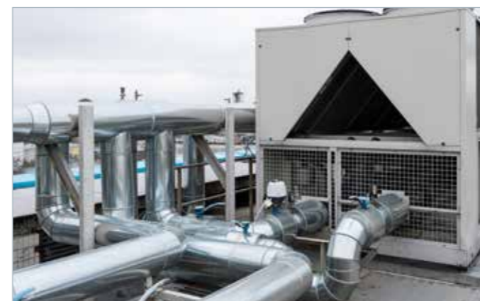
Building cooling systems
