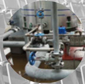
FIRE PROTECTION SYSTEMS
